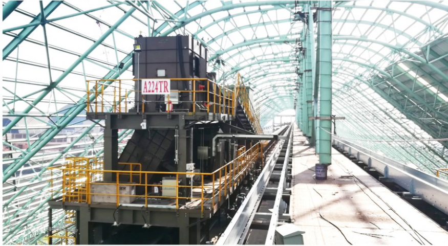
The feeding system in operation at Zhanjiang Steel's new ore yard
