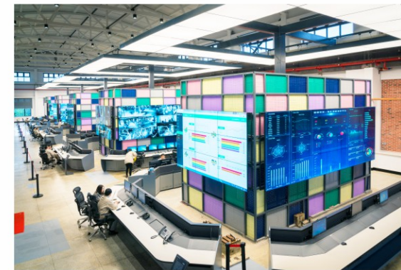
Shaogang's upstream-BF intelligent integrated control centre, built by CISDI on an EPC basis, has now been started up
