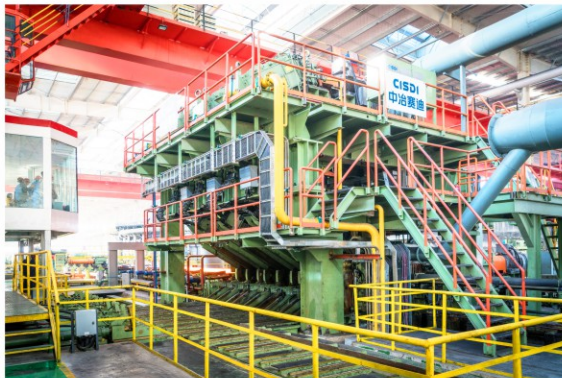
Dalipal's mandrel tube mill during hot-commissioning; the mill was designed and manufactured by CISDI
